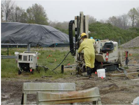
Figure 3: Operator Ramming Drill Steels into the Ground with the GeoProbe. The Grout Pump is Located at the Left of the GeoProbe.
