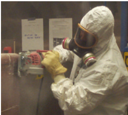
Figure 1. An operator using the Milwaukee Worm Drive Circular Saw to make a horizontal cut.
