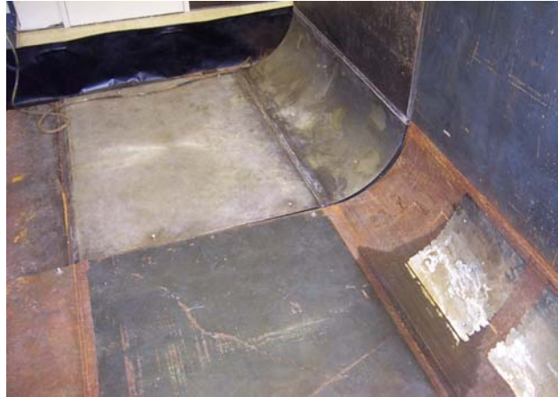
Figure 4: View of the Mockup Tank Interior Illustrating the Knuckle Region for Examination.
