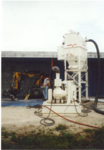
The vacuum extraction system used to capture and collect dust and debris during scabbling.
